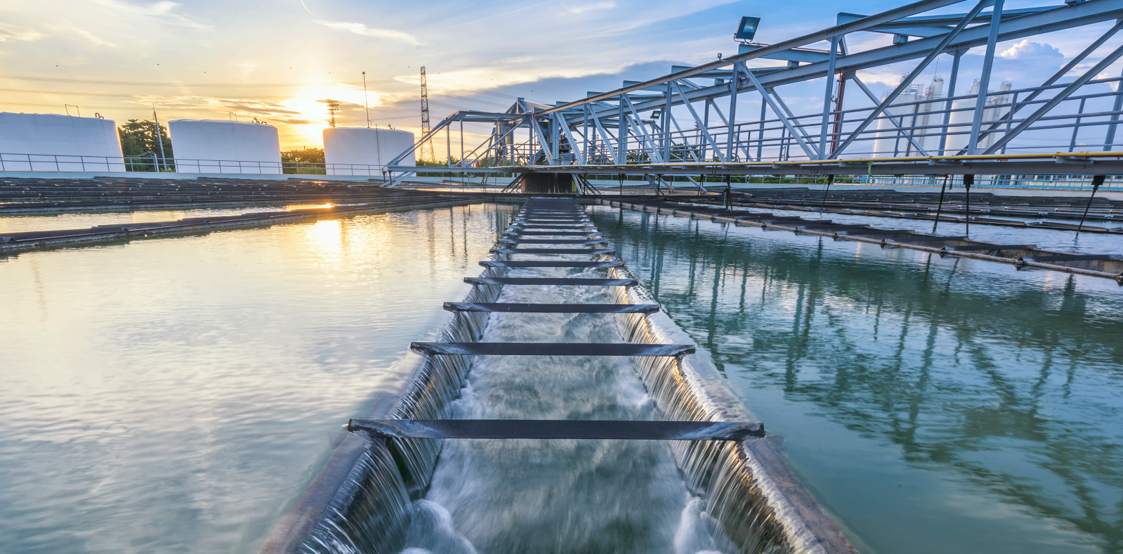
Image caption: Water holding pools at a drinking water plant. Photo from iStock.
